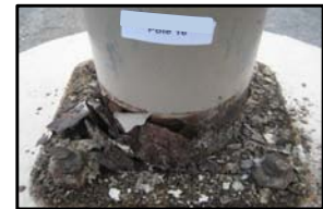
Positive Identification of Dangerous Corrosion
